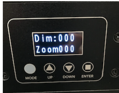
NO DMX CABLE CONNECTED
