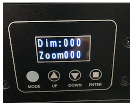
NO DMX CABLE CONNECTED
